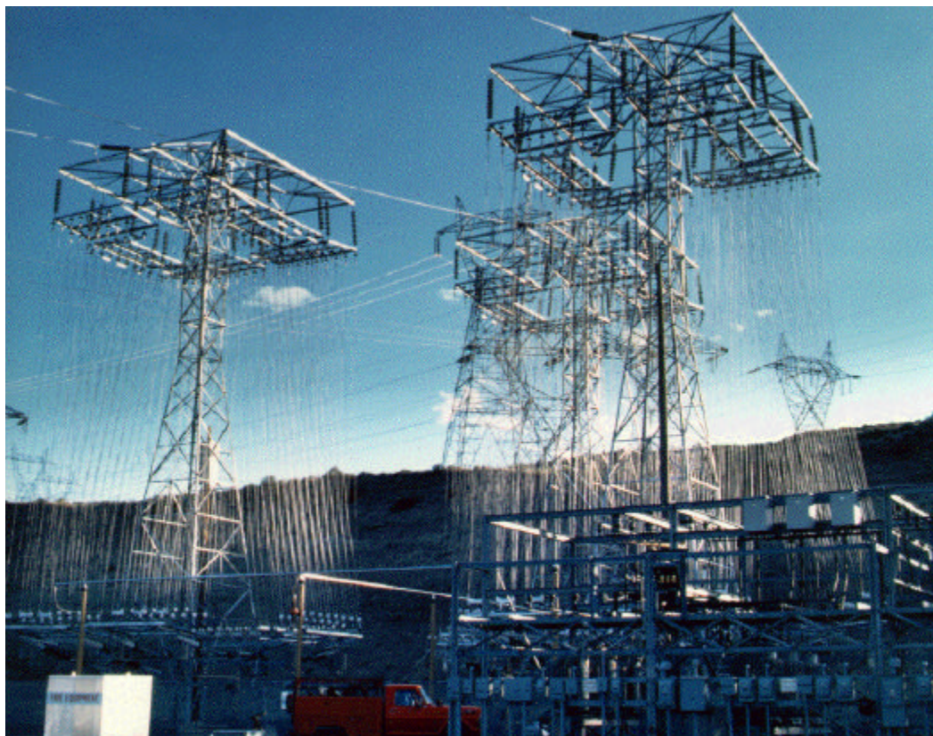
Figure 7-19 The BPA Braking Resistor
